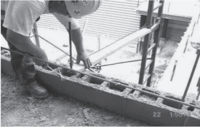
Protection often removed to work
